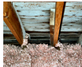
Attic moisture. Vareii
