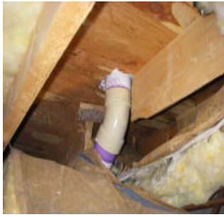
A frequent sight in crawl-spaces.
