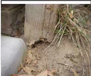
Pressure treated deck supports do rot! J. Cranor
