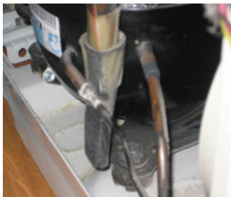
Chinese drywall corroding refrigeration lines on a refrigerator
