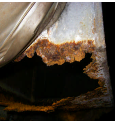
Check metal duct work on or near the crawl space floor. J. Cranor, Glen Allen
