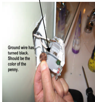
Ground turned black from volatile compounds in drywall. Corrosion increases resistance.
