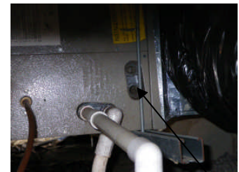
Plug unused drain ports to prevent air leaks. B. Blackwell, Powhatan
