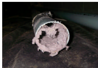
PVC used as dryer vent. J. Cranor, Glen Allen
