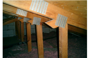
Cut trusses are a common problem! Kenny Hart, Virginia Beach
