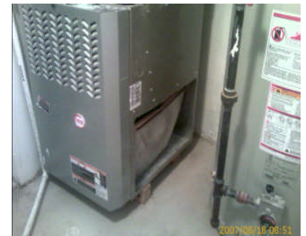
Negative pressure from the furnace return could cause the water heater to back draft. Kenny Hart, VA Beach
