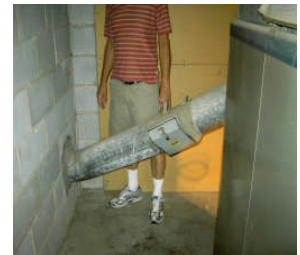
Downward sloping flue pipe. But it was installed this way! Banks Garrison, Abingdon
