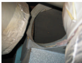
Disconnected return duct pulling air from crawlspace. F. Simmermon, Norfolk
